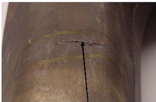
Crack through forward side of tailpipe.
