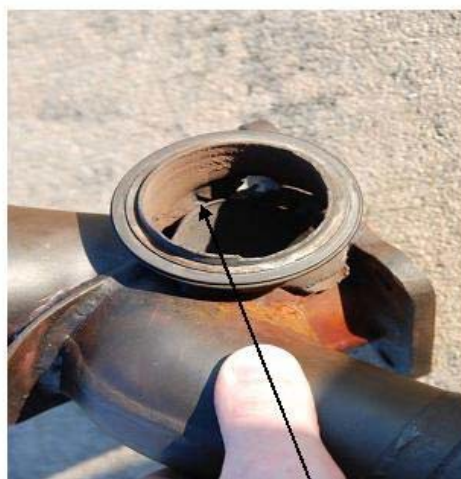
Photo 2: Wye waste-gate elbow attach flange fatigue failure.
