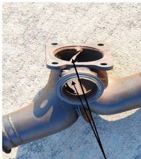
Photo 1: Wye, with failed internal baffle.
